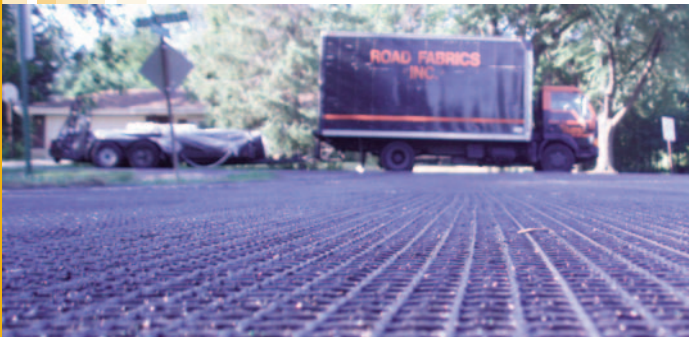
The GlasGrid® System was installed quickly and with minimal inconvenience to residents.
